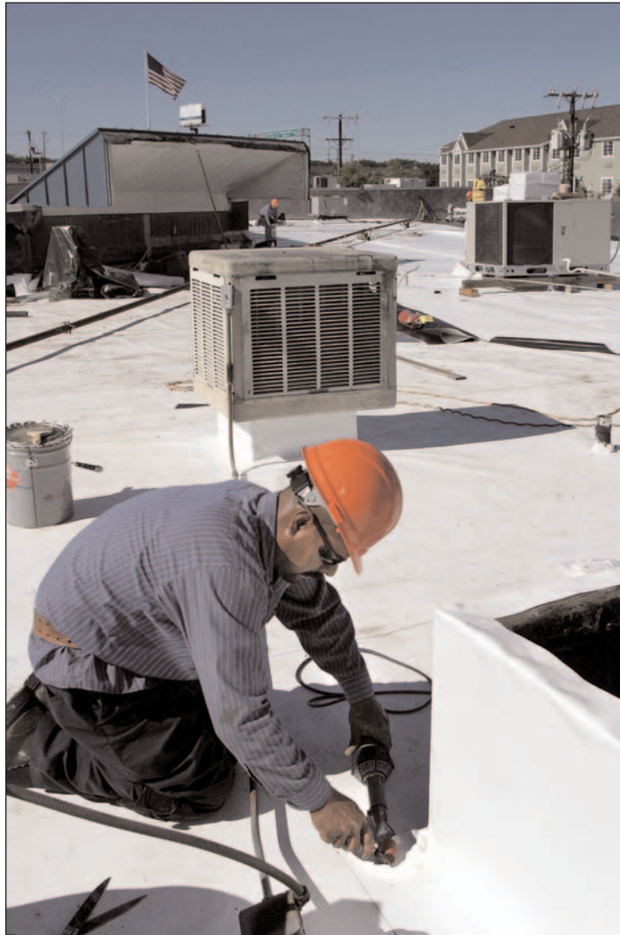
Beldon Roofing’s Ricardo Navarro works on a commercial job. The company started expanding into commercial work in the 1960s. By 1980, residential roofing made up only about 10 percent of its business, said owner Mike Beldon.
